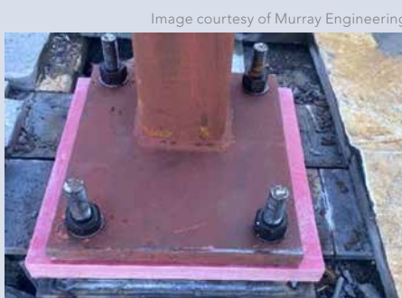
Figure 6. Thermal break pad (pink) used on canopy at Bethany Terrace.
